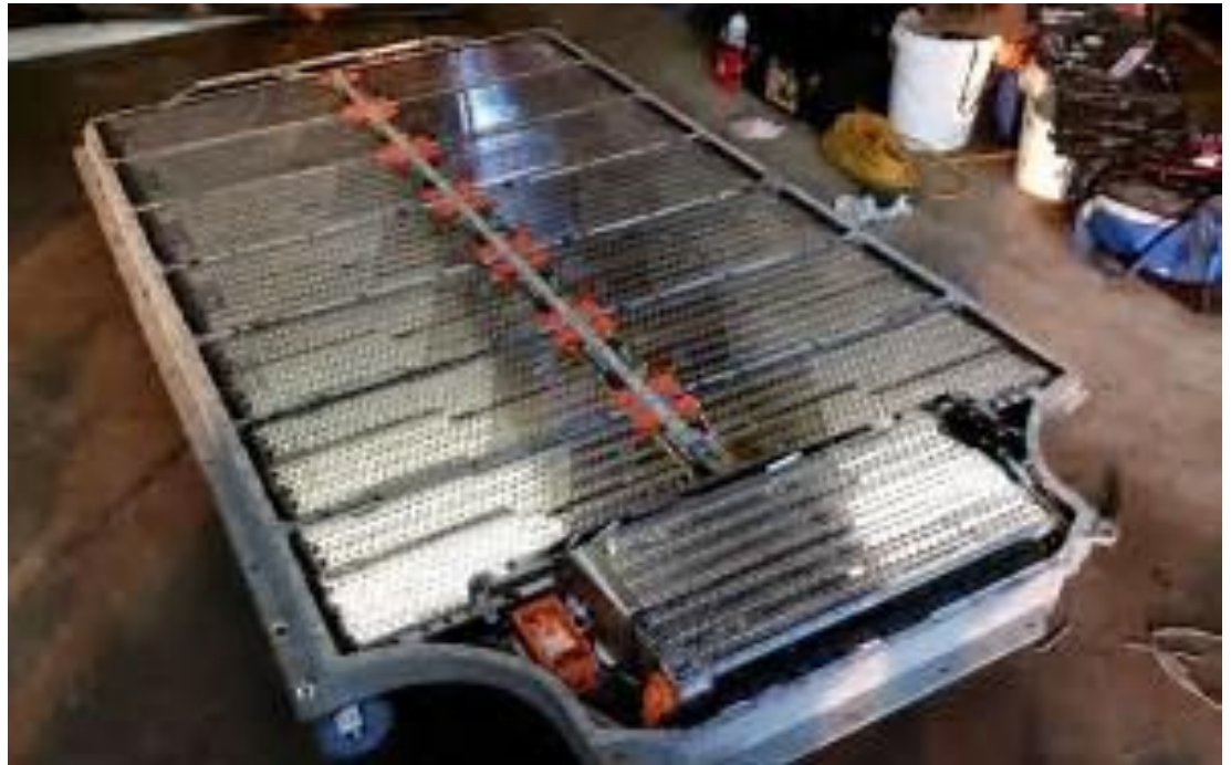
7,000 batteries are installed under body
